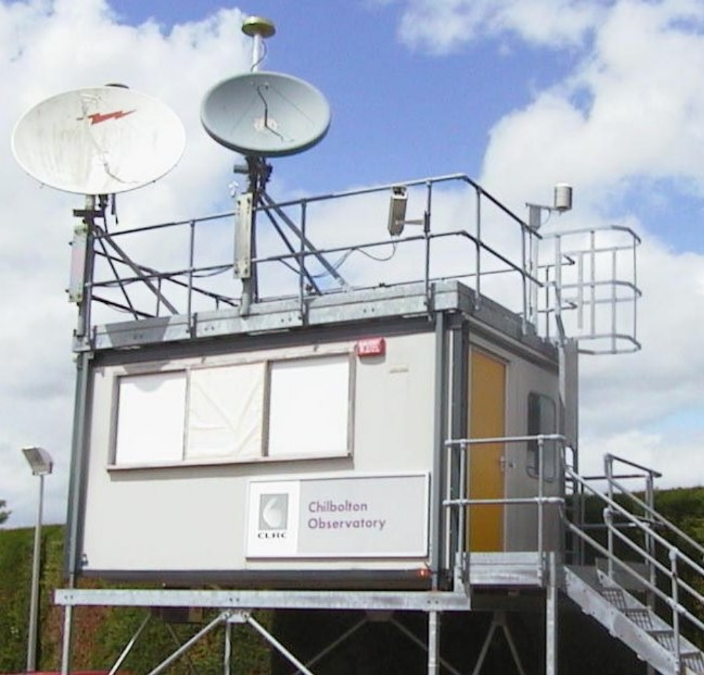
The receive cabin at Sparsholt in Hampshire
